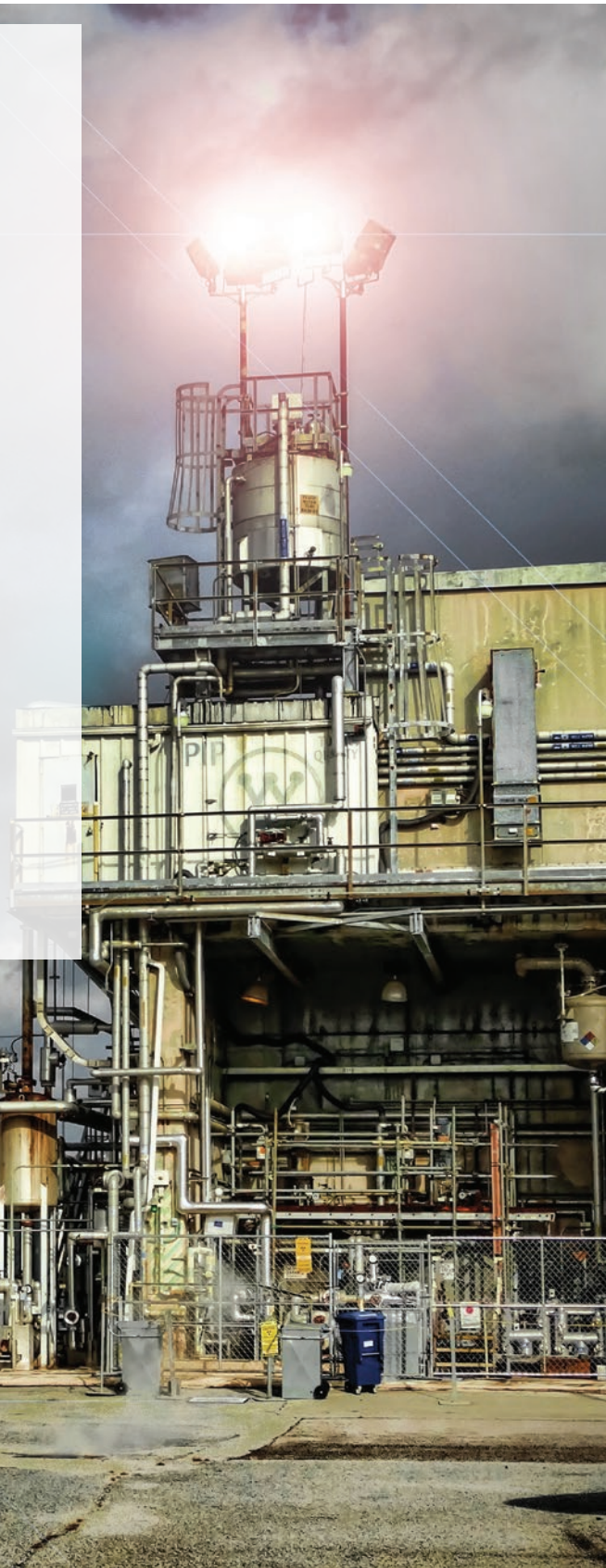
The 2F Evaporator at the Savannah River Site. photo: Savannah River Site Photography
