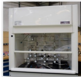
Gas manifold cabinet created at SRNL was shipped to INL and installed.
