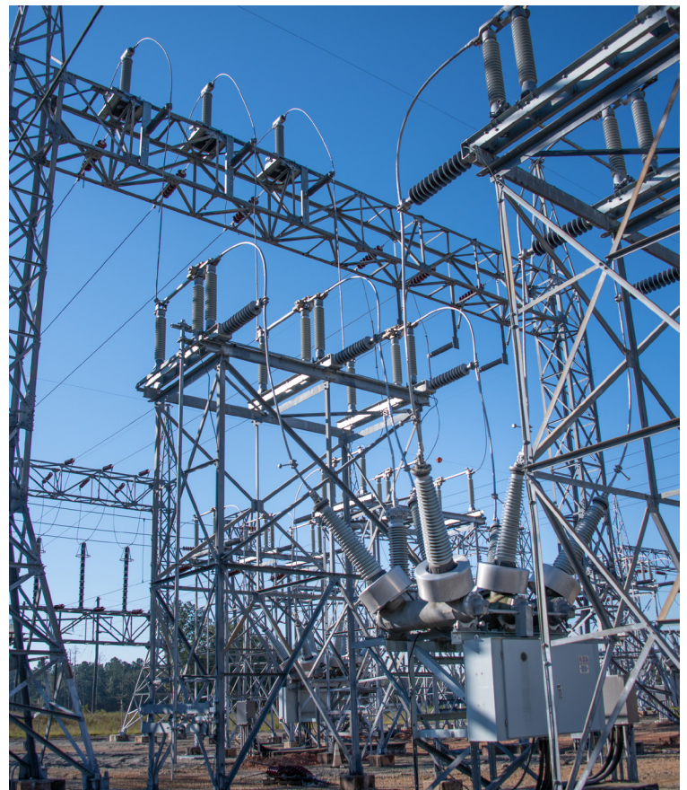
Electric Phenomenon Clusters installed on SRNL transmission network.
