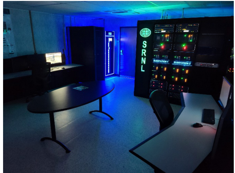
SRNL's Critical Infrastructure, ICS, and Cybersecurity Lab (S-CIIC) located on site at SRS.
